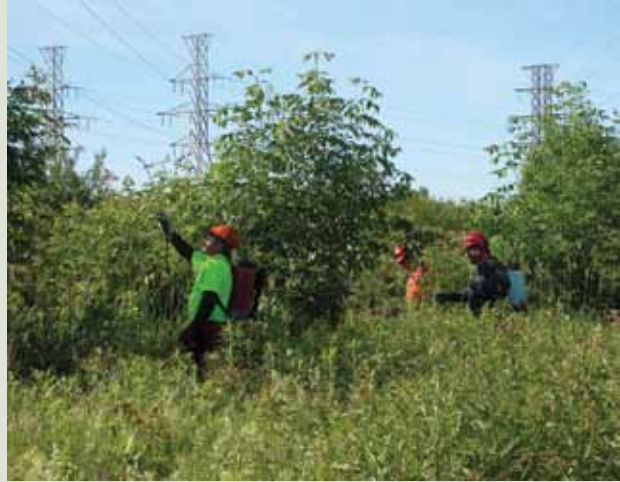
Vegetation on NYPA's ROW is controlled by a variety of methods. Many years of research have shown the lowest-cost, long-term control is accomplished through the judicious use of herbicides, either alone or in a combination of mixtures. Shown here is a crew conducting foliar application on NYPA's ROW.
